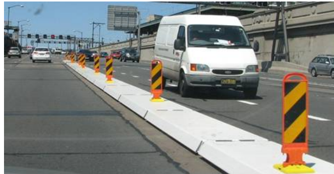
Figure 5.16: Application of Typical Tidal Flow Devices (remotely controlled moveable median)
