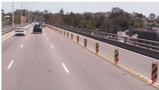
Figure 5.12: Enhanced lane separation devices (Collapsible delineator)
