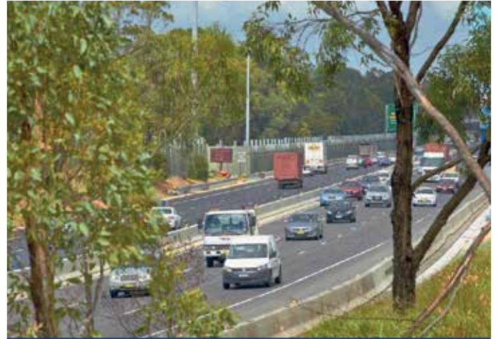
November 2014 near Liverpool, significant progress on the motorway with the project near completion and three lanes open
