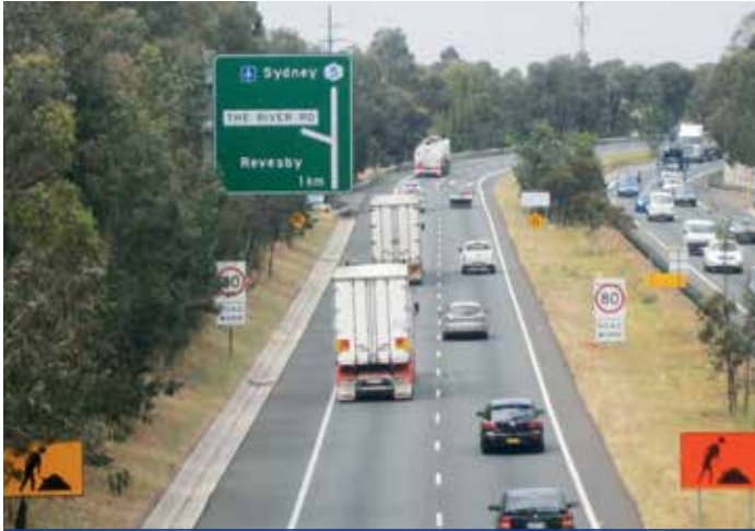
November 2012, early days on the M5 West Widening project, eastbound before The River Road, Revesby
