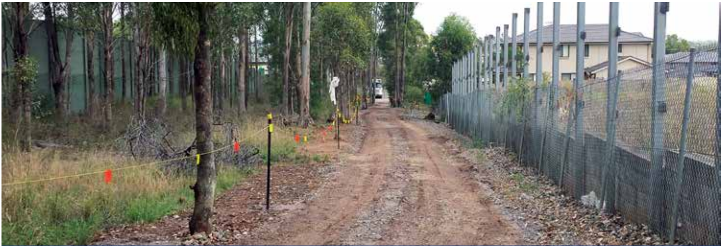
Reduced clearing for the access track for the sediment basin near Beech Road, Prestons
