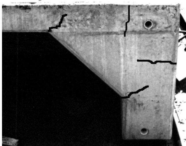
Figure 7.3.5-1 Potential Cracking in Modules
