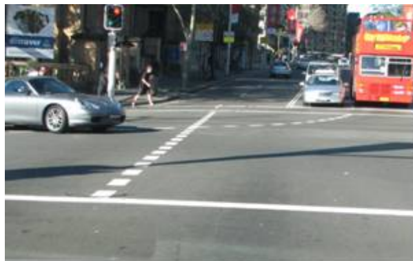
Figure 4.29: Turn Lines at intersection with poor alignment
