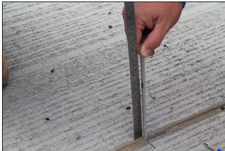
Figure 4. Sealant tab stretched to 100 mm in length above the concrete surface.
