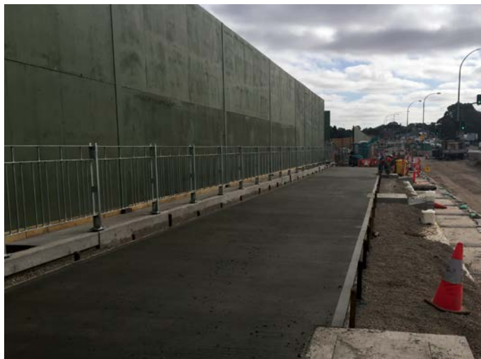
Recent construction progress on the Airport West precinct project at Marsh Street
